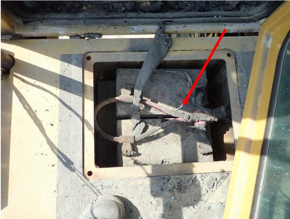
Photo No. 5: Battery box for Trackmobile; inside rear step; no arcing; batteries & connections intact
