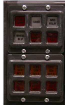
Figure 5-6 – Indicating Lights Panel
