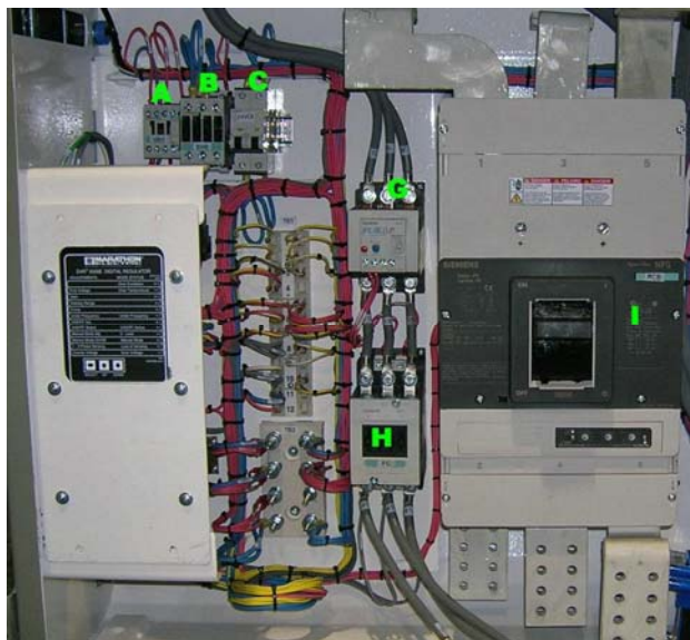
Fig. 7-4 – Circuit Breaker Box
