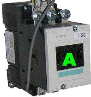
Fig. 5-21 – Load Shed Contactor
